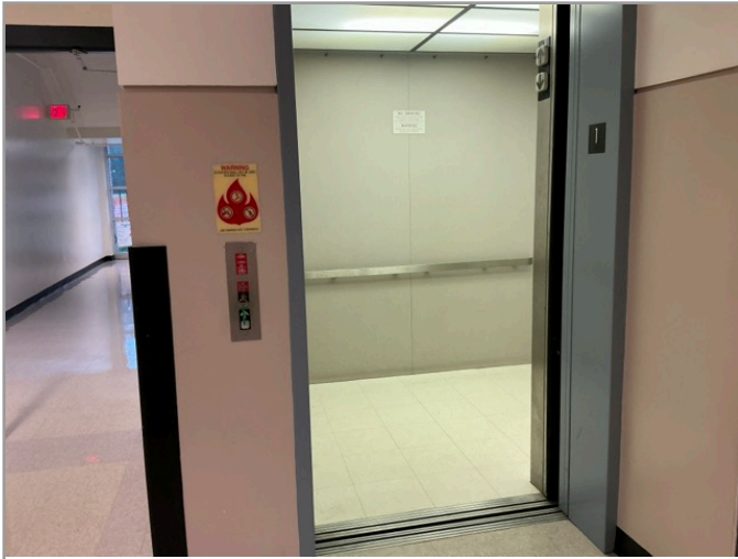
LOBBY LOOKING AT CABS (WITH DOORS OPEN)
