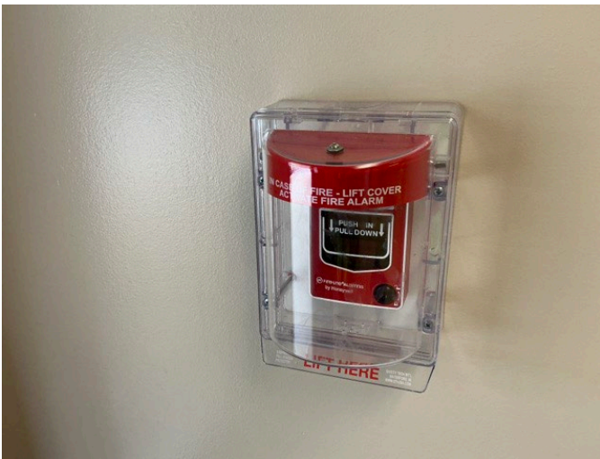
21 - FIRE ALARM PULL STATION
