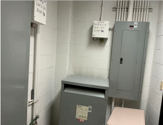
19 - SECONDARY ELECTRICAL ROOM
