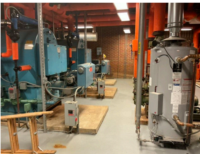
17 - MAIN MECHANICAL ROOM
